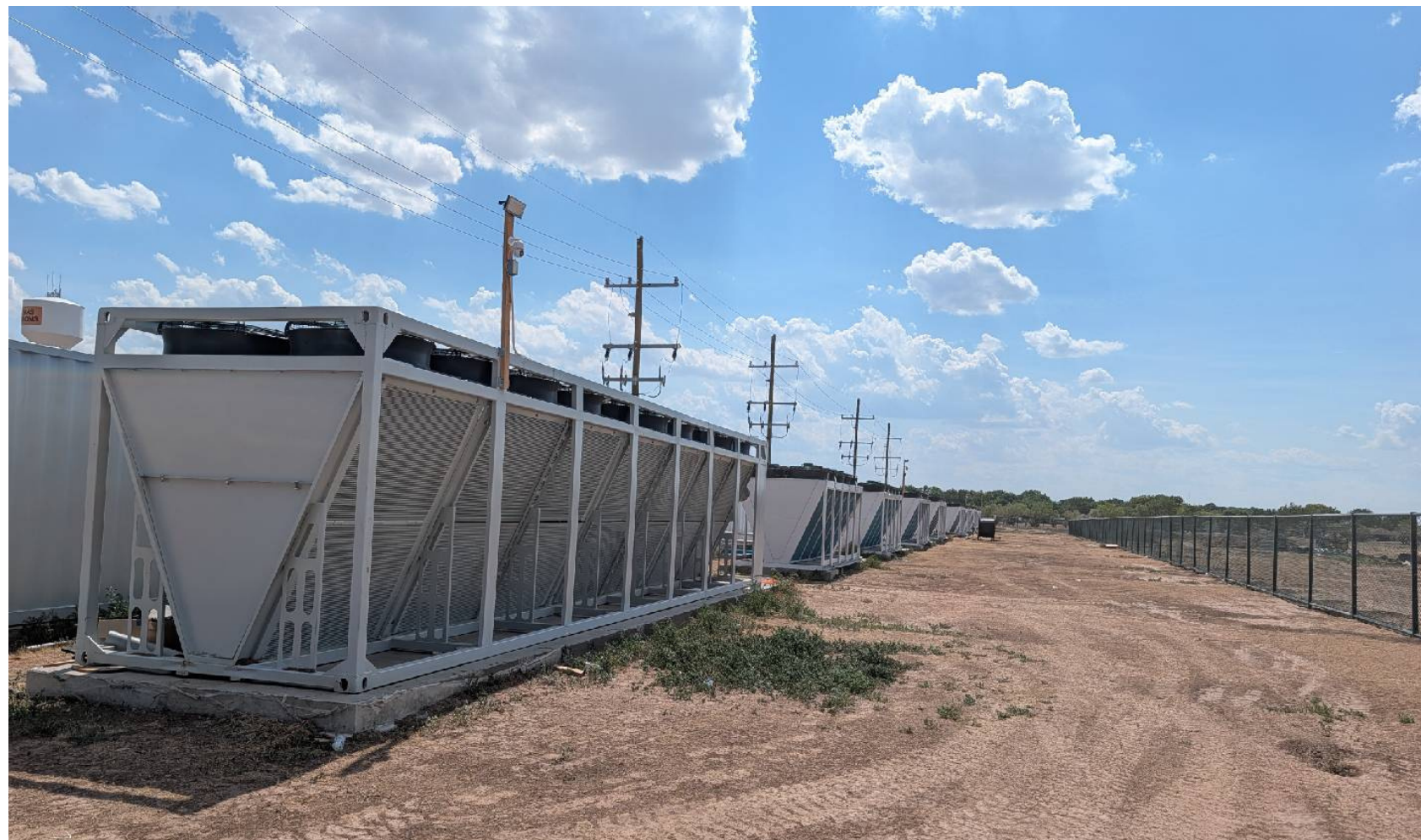
On site today: dry coolers — air only, no spray, no steam, no plume
