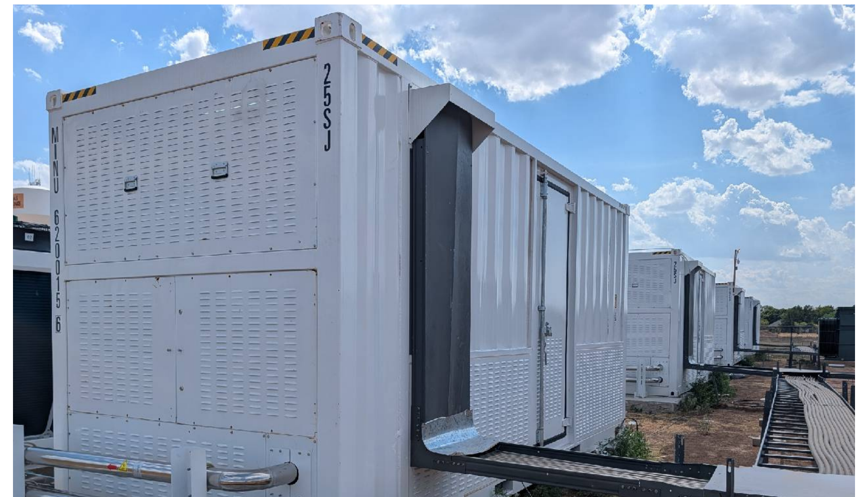
Sealed stainless piping — fixed, welded connections between each container and its cooler
